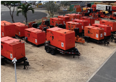
Dri-Prime Pumps for Sewer Bypassing & Dewatering
